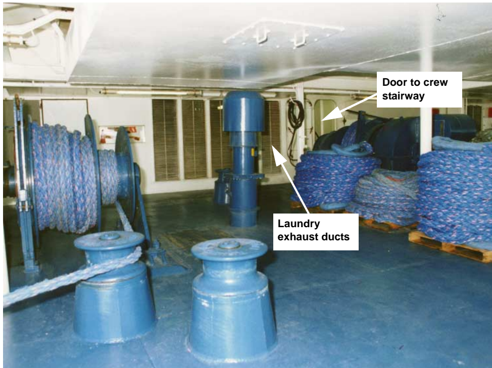
Figure 6a. The ventilation system for the main laundry exhausted onto the mooring deck (shown above), where the synthetic mooring line was spooled on winches or stored on pallets.
