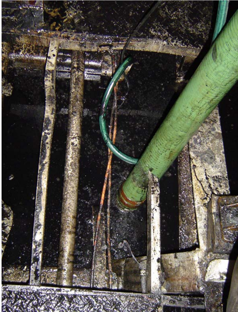
Figure 7. Melted and deformed floor supports and decking next to port inboard engine, looking down. (Large green hose on right and small green garden hose behind it were inserted to control water in bilges after accident; neither was part of vessel's normal equipment.)
